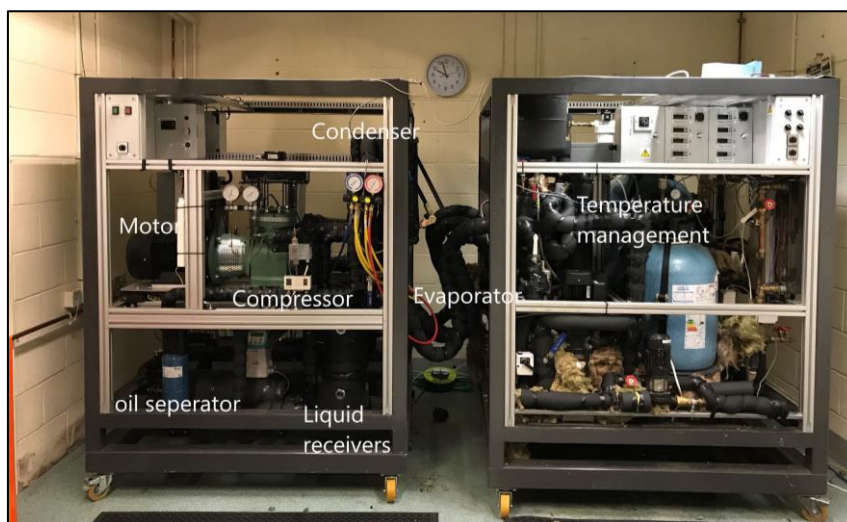
Figure 2 Test-rig development for HTHP
